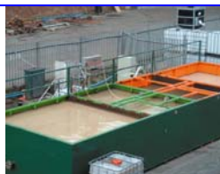
Waste treatment tank
